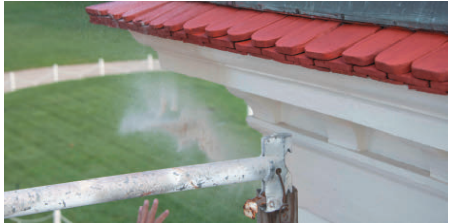
Detail view of painter demonstrating sand-casting on the Mansion's S elevation cornice.
